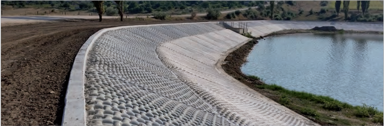
Upper Section with Incomat® Filterpoint C 60.148 and the lower section with Incomat® Crib 10.100 protected lake after installation
